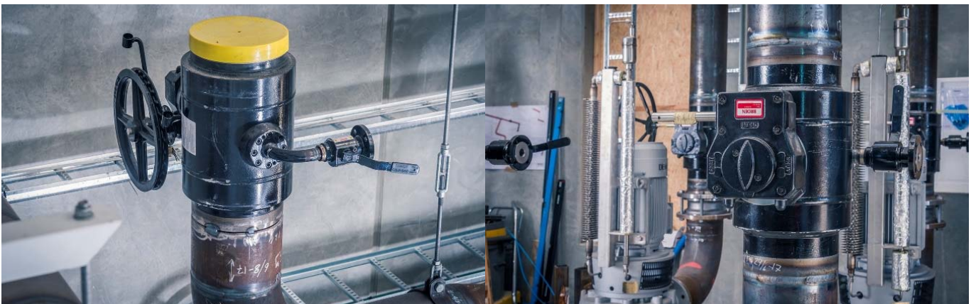
BROEN Ballomax® DN250 – DN400 valves – Double bearing valve balls with Double Block and Bleed and outlet – during welding at Hobro District Heating Station
